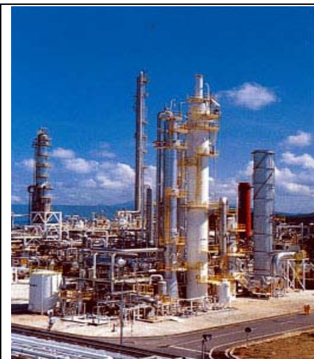
CO 2 Recovery plant in Kedah, Malaysia (160 t/d) (MHI/KEPCO)
